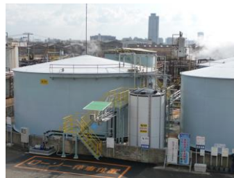
Manufacturing plant of sulfuric acid
