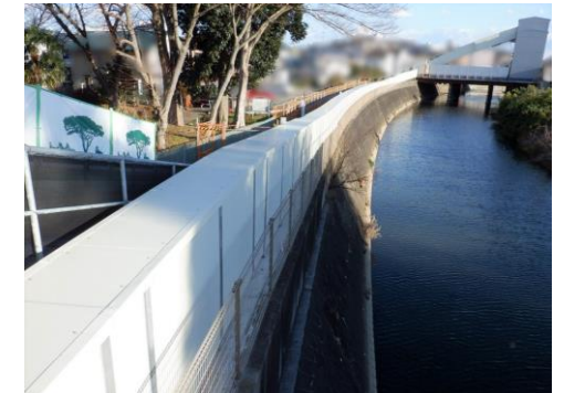
Examples of river flood control (Regulating reservoir construction) Enclosed hanging conveyor (SICON®)
