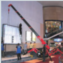
(Mini crawler crane)
