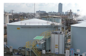
Sulfuric acid tank: Sulfuric acid is an essential basic element for many industries, including chemicals and electronic materials, iron and steel processing, and food processing.
