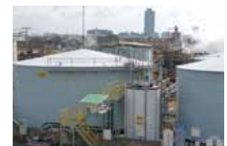
Sulfuric acid production plant
