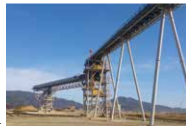
Long-distance belt conveyor
