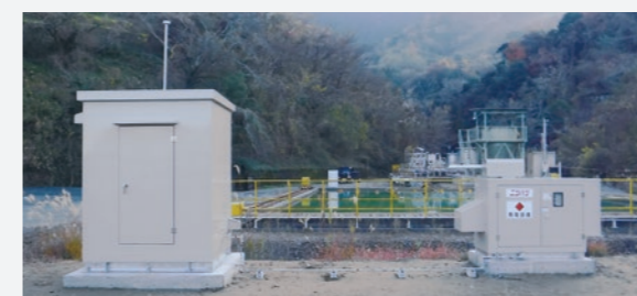
The newly installed emergency generator
