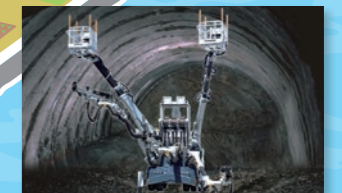
Tunnel drill jumbos These machines are used for the Linear Chuo Shinkansen and other construction projects.
