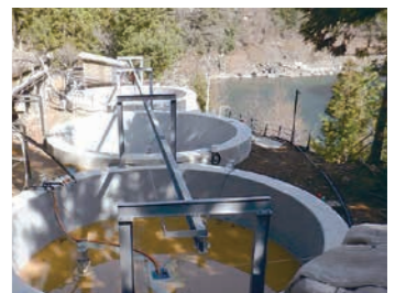
New sludge tanks at the Kune Mine
