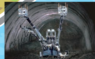
Tunnel drill jumbos These machines are used for the Linear Chuo Shinkansen and other construction projects.
