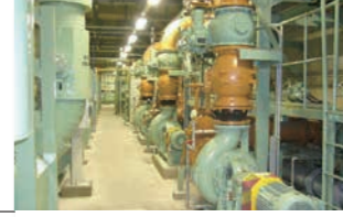
Pumping equipment at wastewater treatment facilities We have a wealth of experience with this equipment at wastewater treatment plants and water treatment plants throughout Japan.
