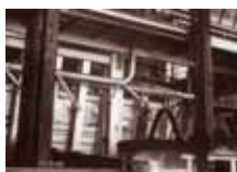
The Furukawa / Outokumpu flash smelting plant.
