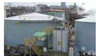
Sulfuric acid production plant
